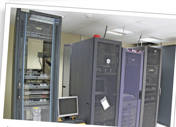
Main Server Sets
